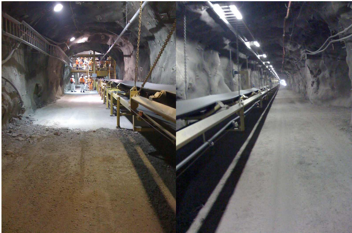
Underground Inclined Conveyor Northparkes Mine
