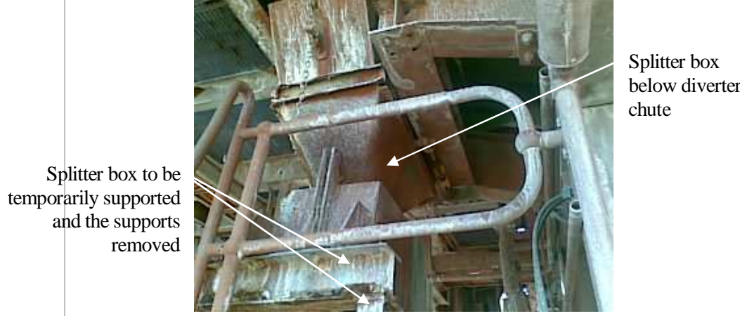
Photo 005 – Splitter box supports
