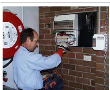
An Installation Inspector tests a distribution sub board. Just part of our commitment to ensure our customer's home and businesses are wired safely.
