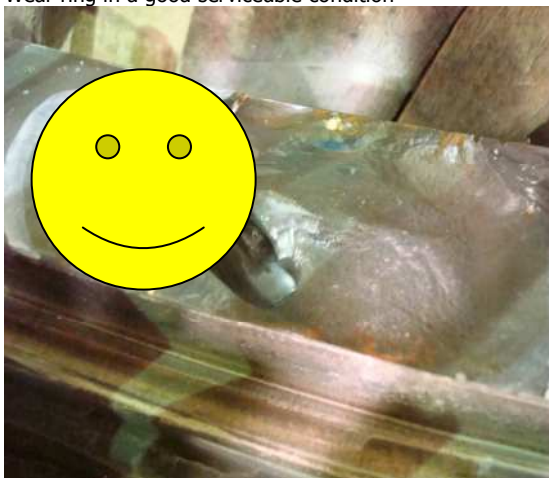
Typical wear of the jet ring due to complete failure of the Wear Ring.
