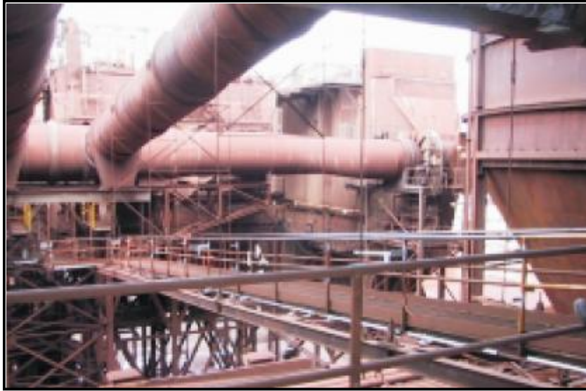
Category V3: Suspended walkway questionable. Needs further investigation.
